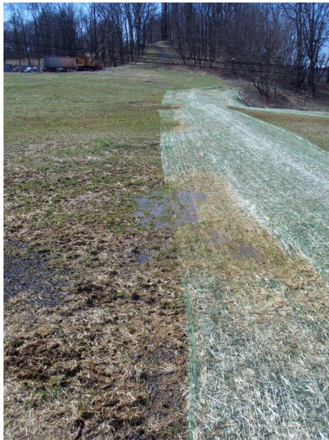
Photo 6 – Areas of ponding noted during second Quarter of LTM-12-2012.
